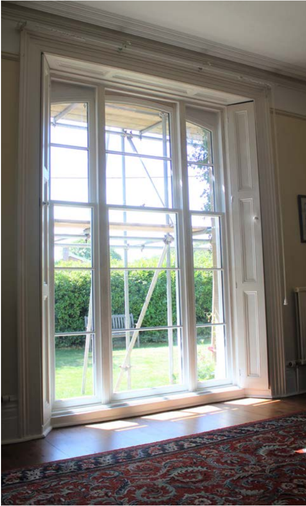
Images of Timber replacement and refurbishment works carried out by our skilled craftsmen
